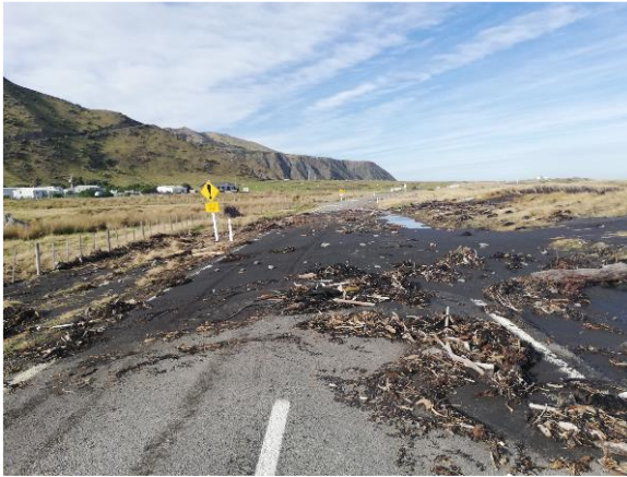
Cape Palliser Rd tidal swell damage
